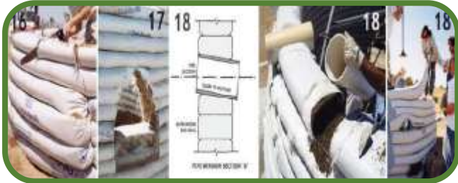
Picture 9: The picture shows the steps of sawing the openings, and placing the ventilation windows in a diagonal way in the outer walls
