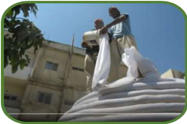
Figure 2 : The construction process by filling the bags .with soil immediately, that is, during construction Source: by researcher
