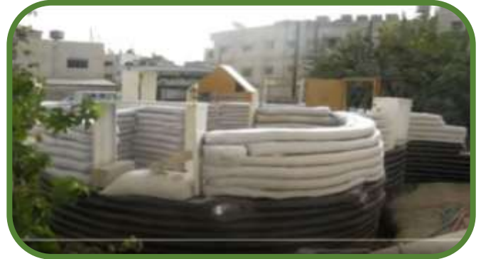
Figure 3: The courses of sandbags are arranged on top of each other and around the openings
