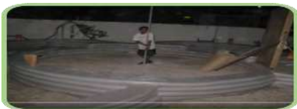
Figure 1 : the circular foundations of the house are made of plastic bafs filled with sand , source : by researcher
